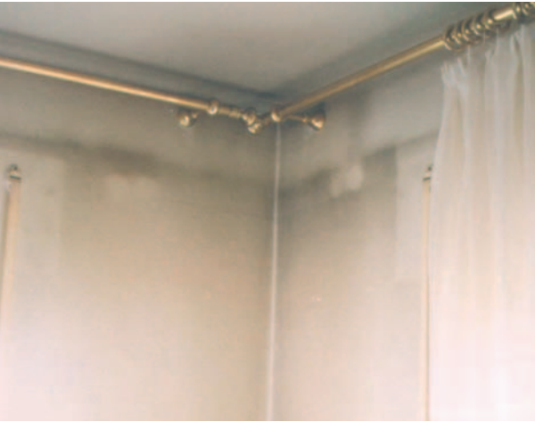
The black film appeared in this room six months after it had been decorated.
