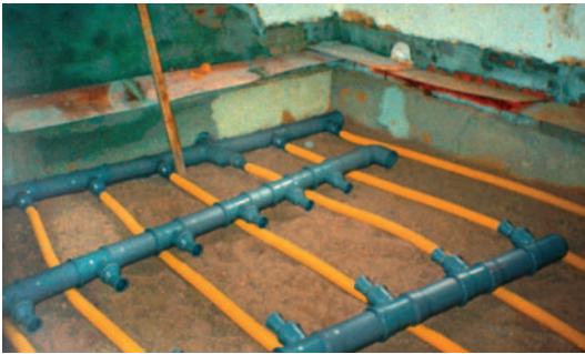
Installation of a drainage system beneath the foundations (here during the construction of the building) with the aim of extracting soil air containing radon and venting it out of the building.
