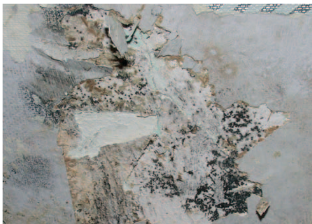
Mould infestation behind wallpaper
