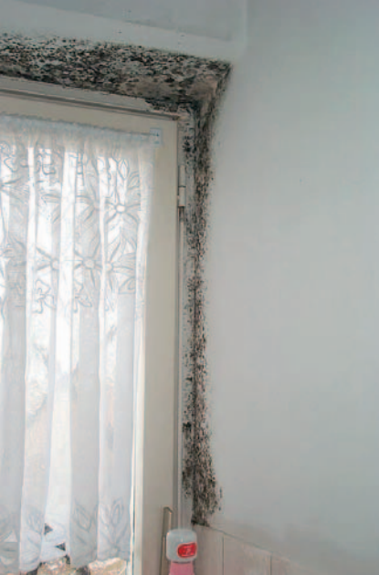
Mould infestation after water damage. Mould fungi are not only an aesthetic problem but also a health risk!
